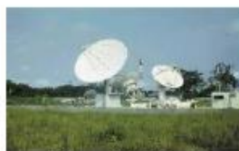
Libreville Fixed Ground Station
